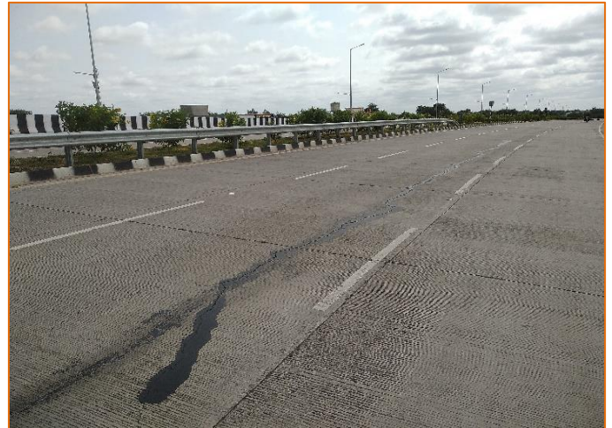
Pavement Condition at km. 287+700 (RHS)
