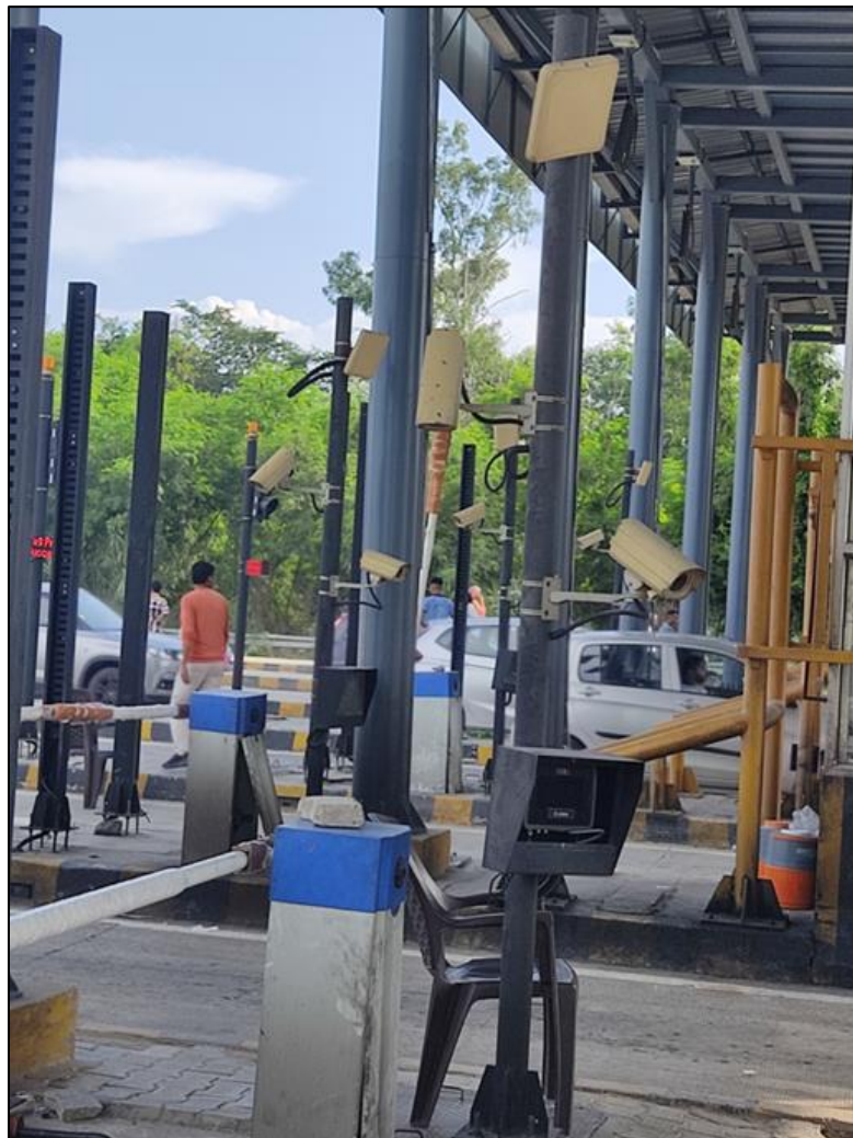
Figure 9-3 RFID ETC Transceiver installed on pole
