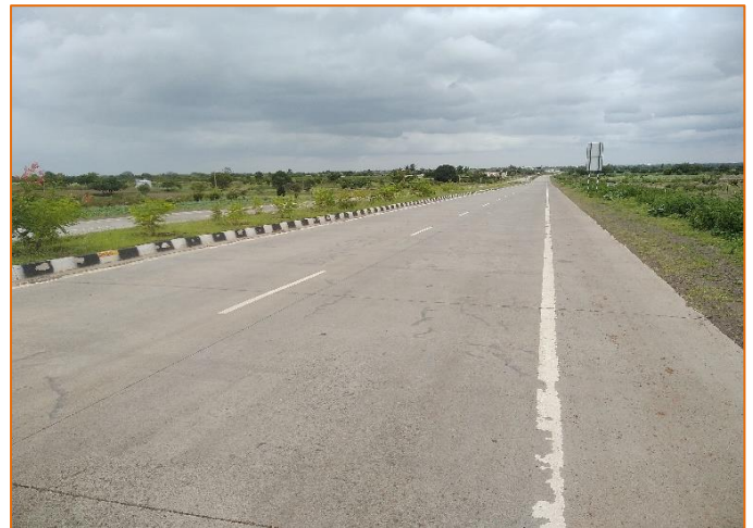
Pavement Condition at km. 319+100 (RHS)
