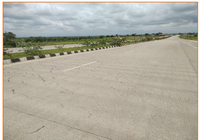
Pavement Condition at km. 304+600 (LHS)
