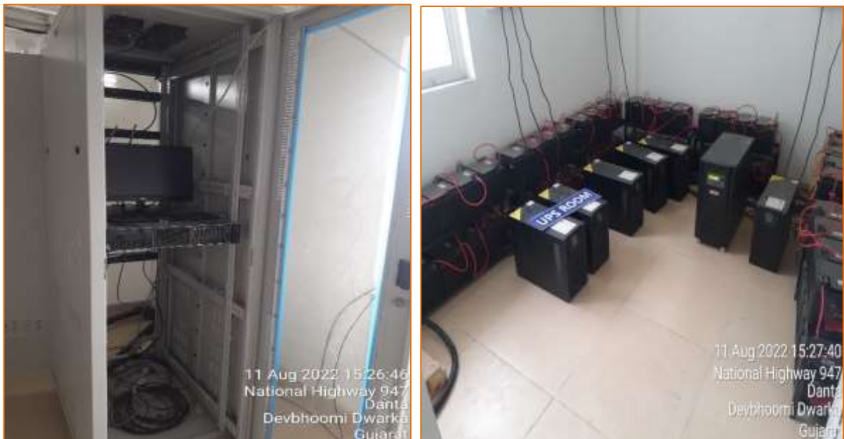
Figure 8-8 Control Room Equipment - Server & Switch rack/UPS Room
