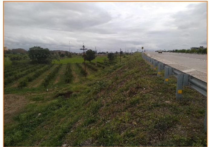
Crash Barrier at High Embankment Location
