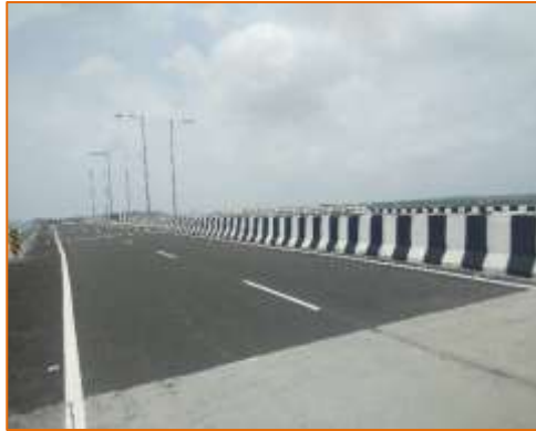
Wearing Coat of ROB at km. 0+527 (RHS)
