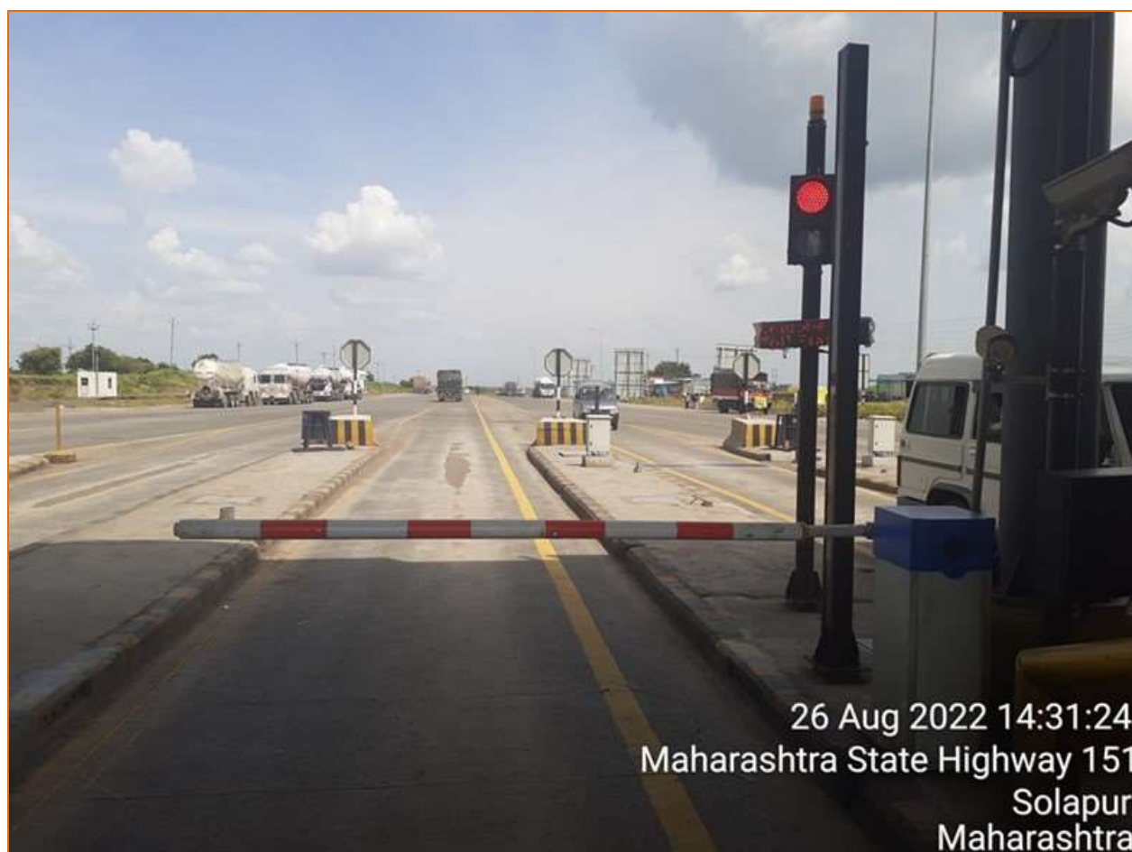
Figure 9-4 Automatic Lane Barrier
