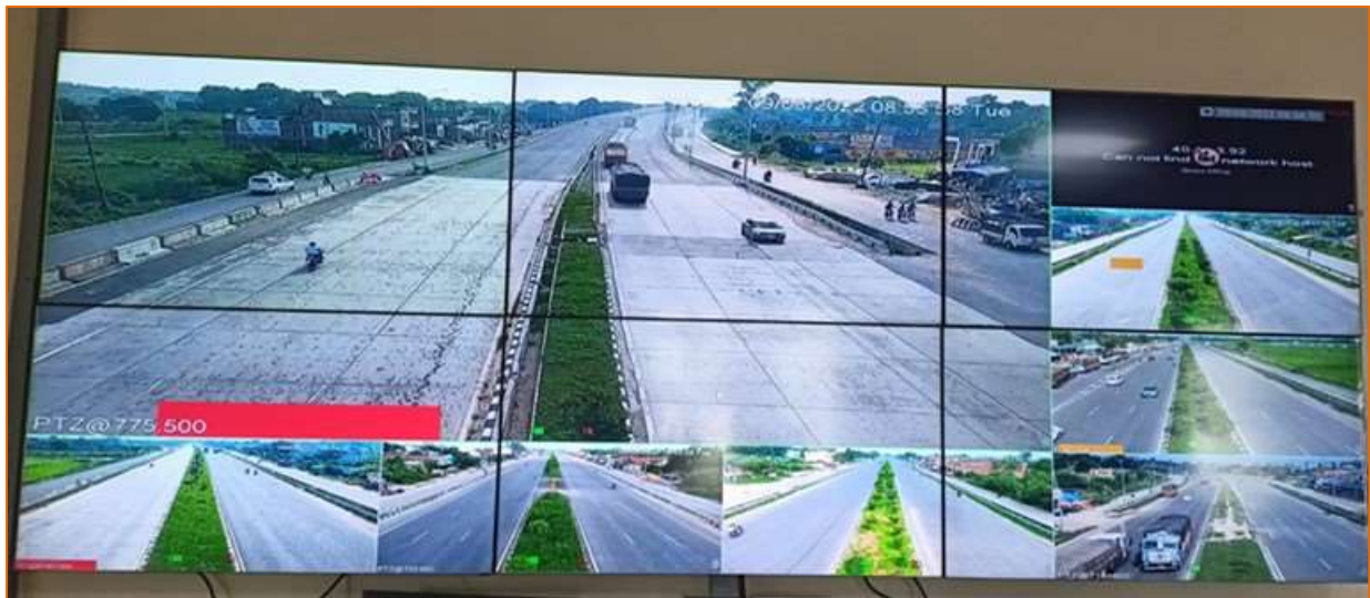
Figure 9-10 Video wall in ATMS control centre
