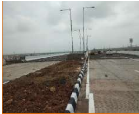
Wearing Coat of VUP at km. 12+420 (BHS)
