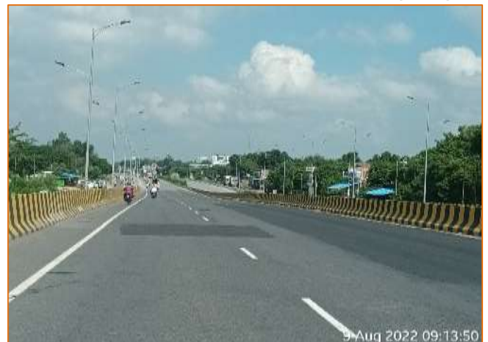
Pavement Condition at km. 779+600 (RHS)
