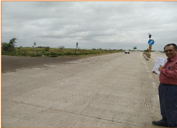
Pavement Condition at km. 306+500 (LHS)
