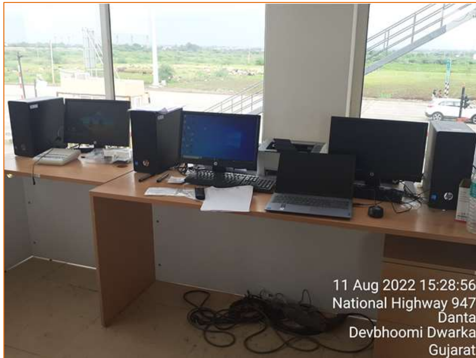
Figure 8-10 Workstations at Control room
