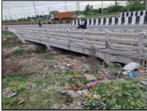
Minor Bridge at km. 77+613 opening blocked (Structure View)
