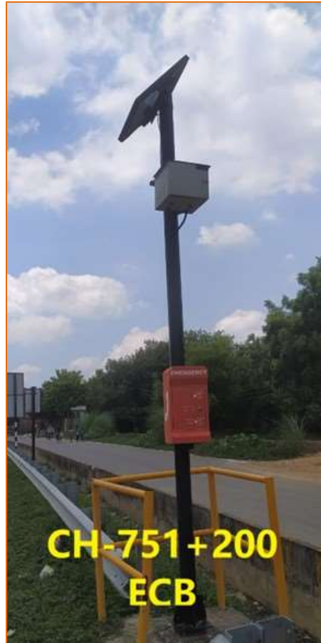
Figure 9-6 ECB at km. 751.200
