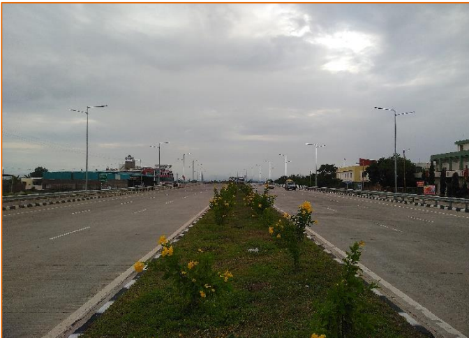
Pavement Condition at km. 285+750 (BHS)
