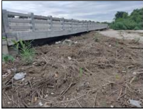
Minor Bridge at km. 72+134 opening blocked (Structure View)
