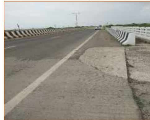
Side View of Minor Bridge at km. 459+038 (LHS) - New - Approach settled
