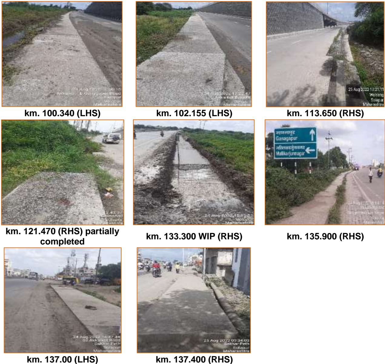
Figure 3-7 Photographs of Drains provided
