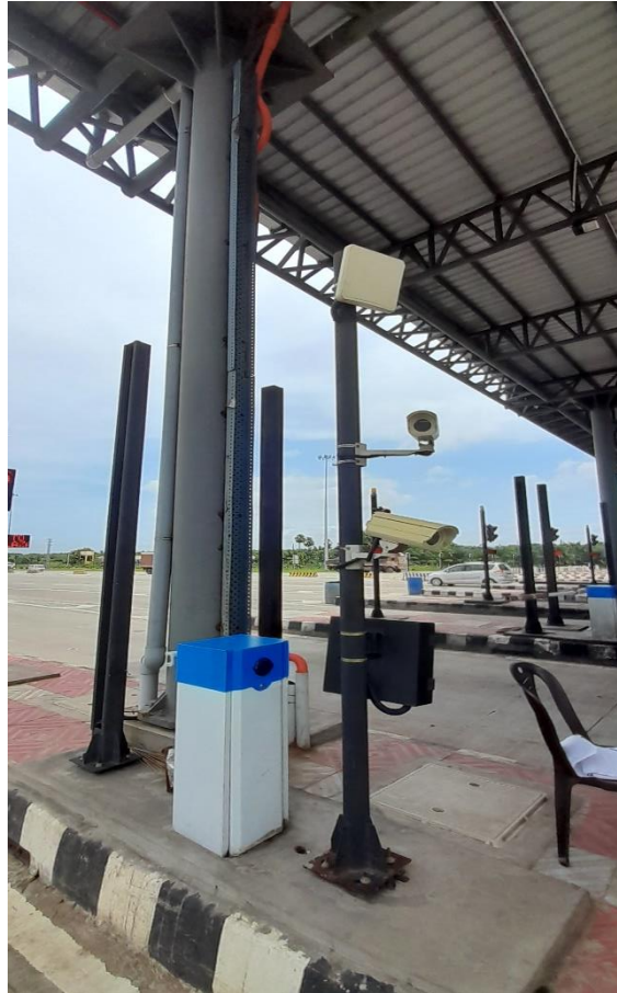
Figure 9-2 RFID ETC Transceiver installed on pole
