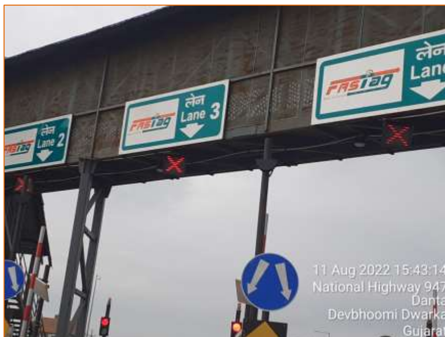
Figure 8-5 Over Head Lane Signal (OHLs)
