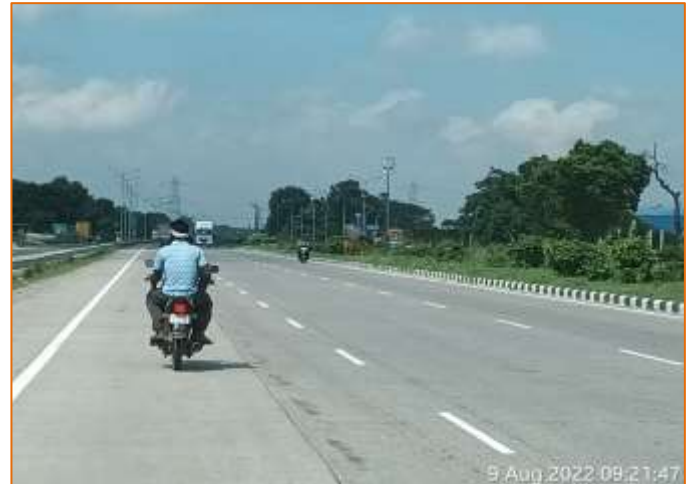
Pavement Condition at km. 785+650 (RHS)
