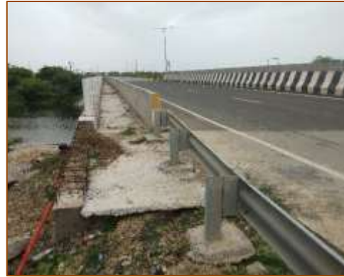
Return wall beam pending of MNB at km. 456+533 (RHS)
