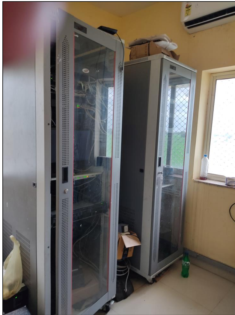
Figure 9-13 Control Room Equipment - Server & Switch rack
