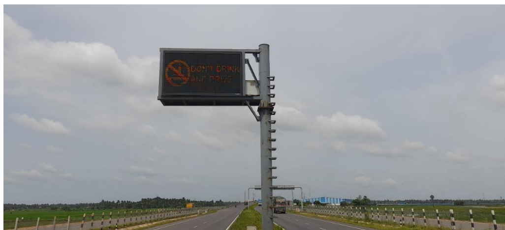
Figure 9-16 VMS on project highway
