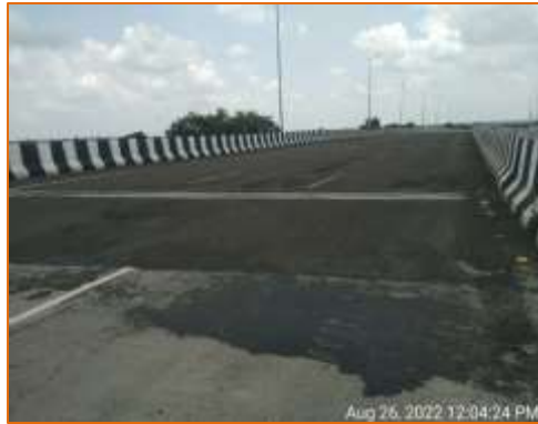
Roughened BC surface of Flyover at km. 103.801 (RHS)
