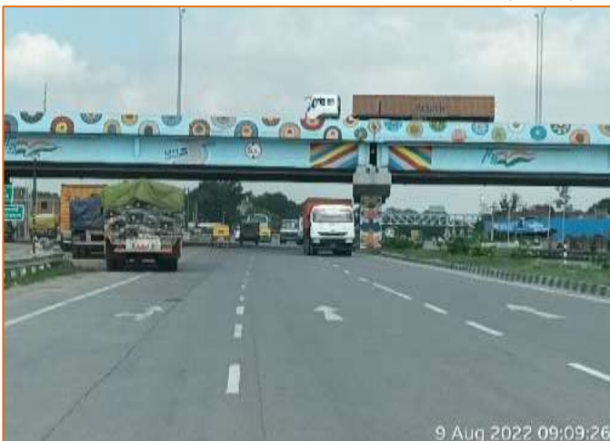
Pavement Condition at km. 782+500 (RHS)
