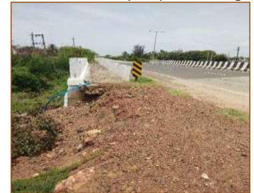
Side View of Minor Bridge at km. 440+350 (LHS) - Rain cut developed
