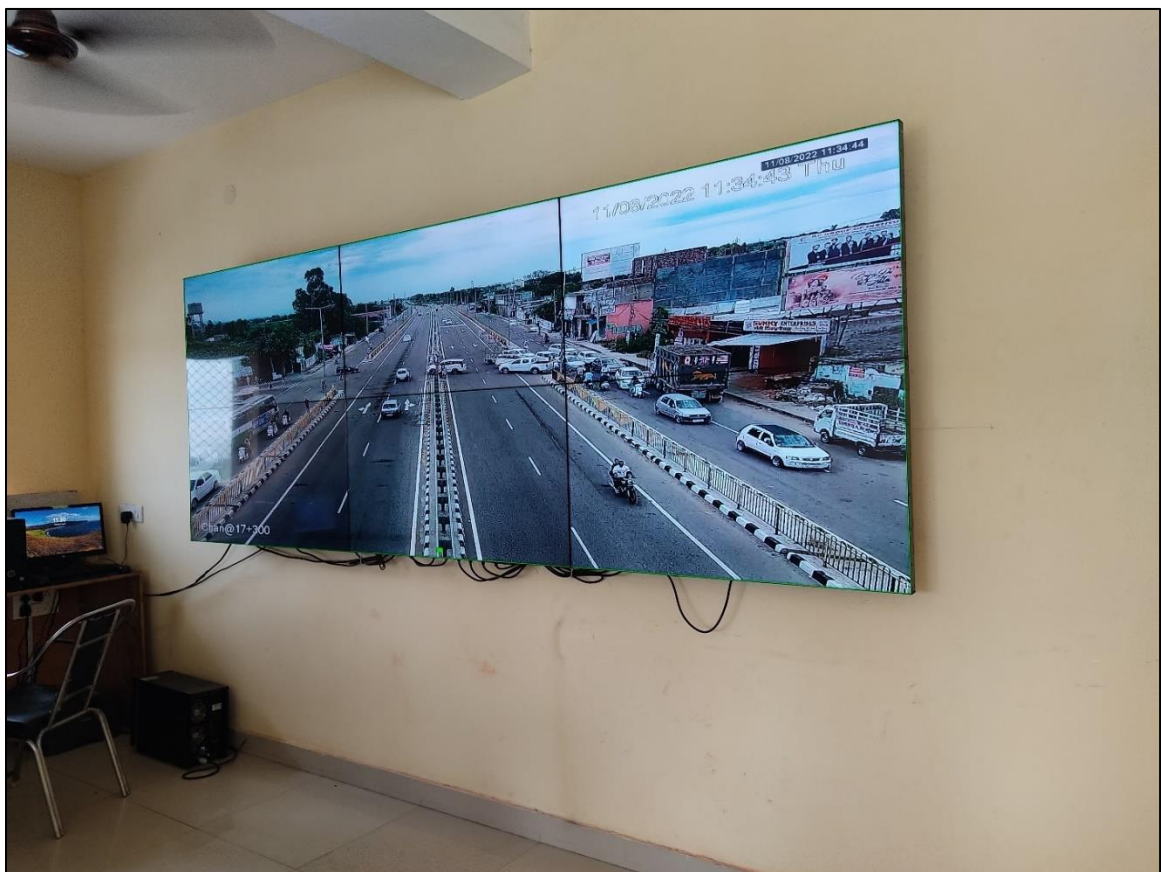
Figure 9-18 Video wall at HTMS Control room
