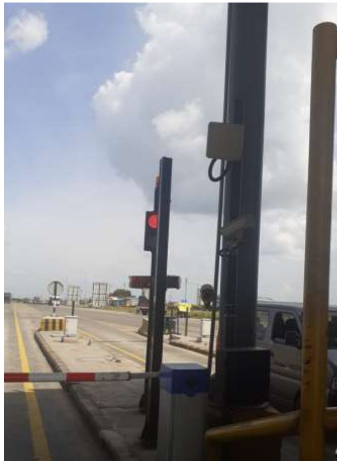
Figure 9-2 RFID ETC Reader mounted on Pole
