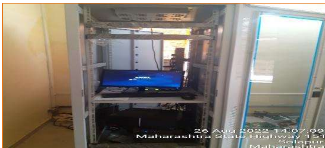
Figure 9-8 Medium Control Room Equipment – Server & Switch rack
