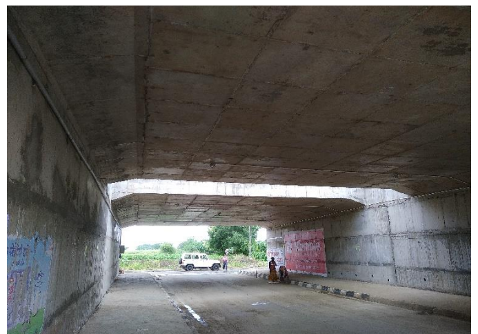
Lighting arrangement made under structures
