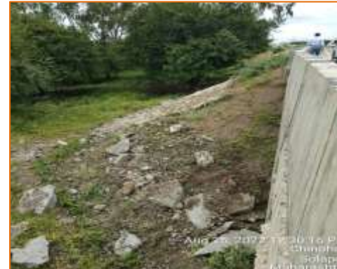
Rubble pitching pending @ A1 side of MNB at km. 124.337 (RHS)
