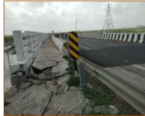
Side View of Minor Bridge at km. 492+030 (RHS) - New - Footpath damaged
