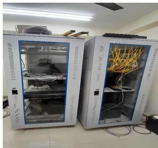
Figure 9-12 Control Room Equipment - Server & Switch rack
