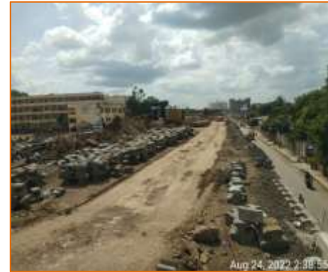
Filling work & RE Block erection work of Flyover is in progress at km. 136.857 @ Akkalkot side (RHS)
