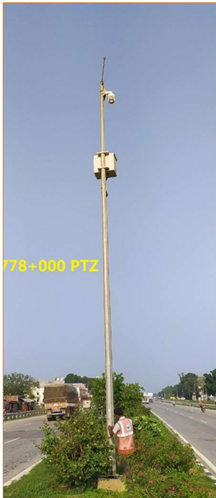
Figure 9-9 PTZ camera at km. 778.000
